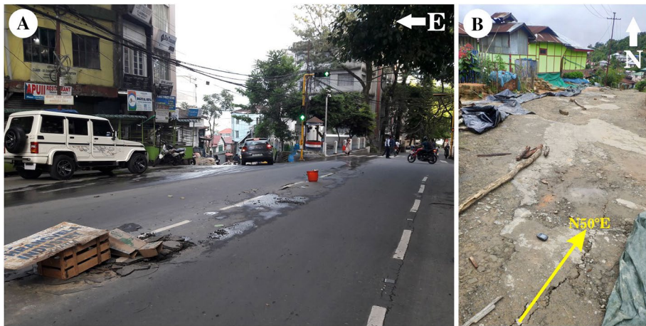
Fig. 3 a Fracture/Cracks developed along the main road near Aizawl District Collector office (trend of fracture: 150^{\circ} ) due to the 21st June 2020, Mw 5.1 earthquake, Aizawl earthquake; b Prominent fractures occurred during the Champhai Earthquake (trend of fracture: 050^{\circ} )
